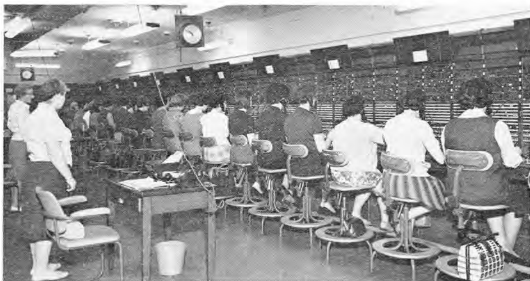
The old and the new. On the left, a large manual exchange (installed at Old Admiralty Building, Whitehall, in 1937 and still in use) and on the right, a section of the apparatus room in an automatic exchange (Rear Admiral R. C. Paige at the opening of the new Portsmouth Dockyard Exchange in 1966.)
